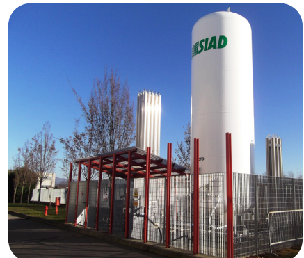
High Pressure System for Gas Testing
