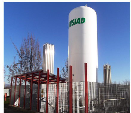
High Pressure System for Gas Testing
